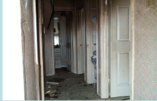
Fire room, first door to the left (cannot see in this photo). Door at end of hall is where Engine 6 Firefighter advanced. Engine 6 LT advanced into room on the right.
